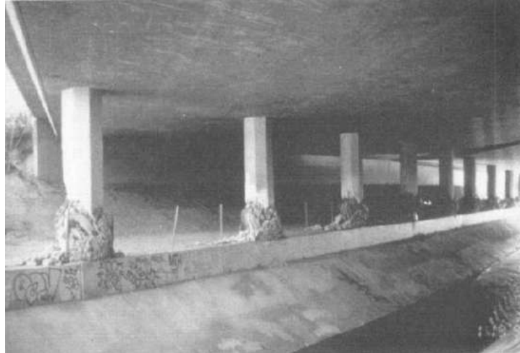
Figure 2.5. Compression failure and bulging of piers along bent 3. Bull Creek Canyon Channel Bridge. Photograph courtesy of Earthquake Engineering Research Institute (Papazoglou and Elnashai 1996).
