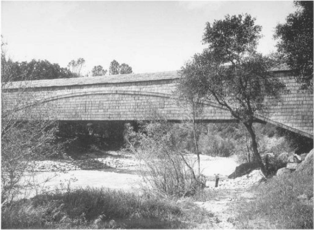
FIGURE 67.4 The Bridgeport Covered Bridge in California may be the longest single-span, 70.1 m, covered bridge in the world. The superstructure is a Burr arch superimposed on a Howe truss. It was a toll bridge built by David Wood in 1862, and was later purchased by the Virginia Turnpike Company. (Courtesy of California Department of Transportation.)
