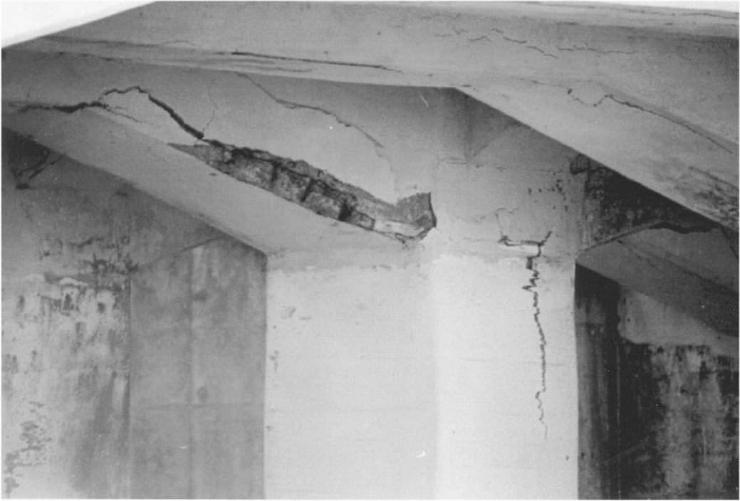
FIGURE 65.20 A typical reinforced concrete bridge damaged by corrosion.
