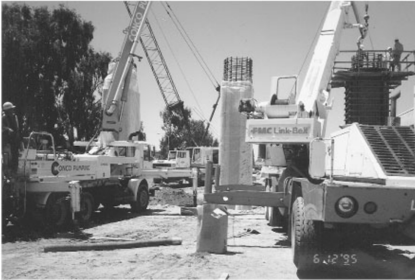
FIGURE 48.2 Crane used to hold the column cage; column is being cured with plastic wrap.
