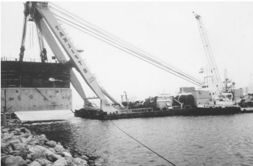
FIGURE 47.29 Lifting box caisson from quay wall on which it was prefabricated and transporting it to site while suspended from crane barge.
