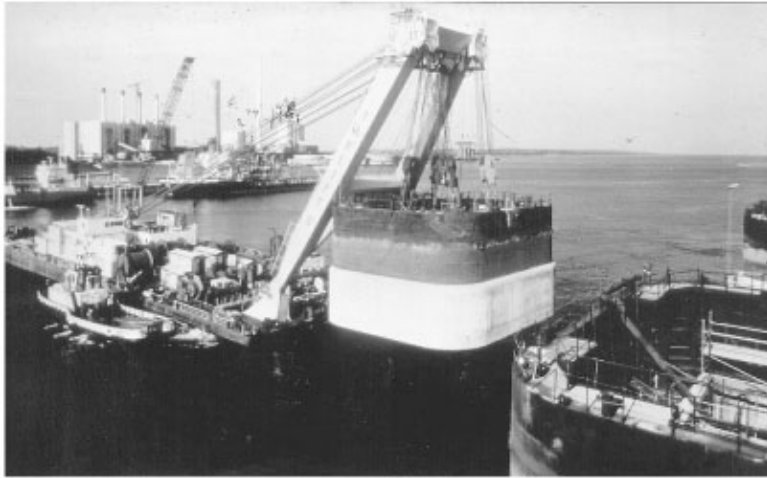
FIGURE 47.30 Setting prefabricated box caisson on which is mounted a temporary cofferdam, Great Belt Eastern Bridge, Denmark.
