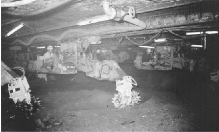
FIGURE 47.17 Excavating within pressurized working chamber of pneumatic caisson for Rainbow Suspension Bridge, Tokyo. (Photo courtesy of Shiraishi Corporation.)
