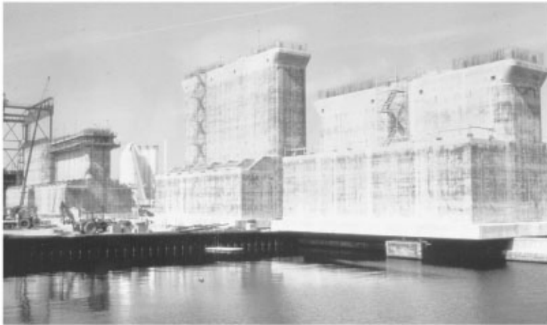
FIGURE 47.22 Prefabricated concrete box caissons are moved by jacks onto pier for load-out.
