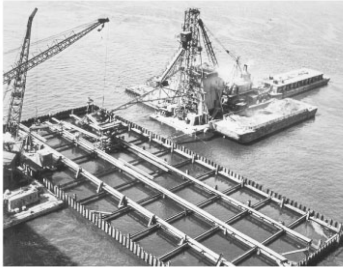
FIGURE 47.9 Large steel sheet pile cofferdam for Second Delaware Memorial Bridge, showing bracing frames.
