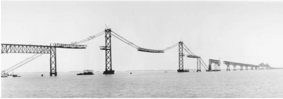
Figure 45.6 Suspension spans of first Chesapeake Bay Bridge, Maryland, 1952. Deck steelwork is under erection and is about 50% complete. A typical four-panel through-truss deck section, weighing about 100 tons, is being picked in west side span, and also in east side span in distance. Main span is 1600 ft (488 m) and side spans are 661 ft (201 m); towers are 324 ft (99 m) high. Cables are 14 in. (356 mm) in diameter and are made up of 61 helical bridge strands each (see Figure 45.8 ).
