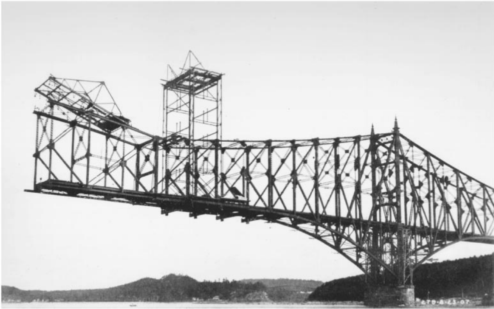
Figure 45.11 First Quebec railway cantilever bridge, 23 August 1907. Cantilever erection of south main span, six days before collapse. The tower traveler erected the anchor span (on falsework) and then the cantilever arm; then erected the top-chord traveler, which is shown erecting suspended span at end of cantilever arm. The main span of 1800 ft (549 m) was the world's longest of any type. The sidespan bottom chords second from pier (arrow) failed in compression because latticing connecting chord corner angles was deficient under secondary bending conditions.
