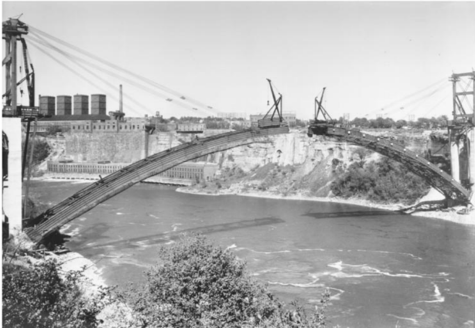
Figure 45.2 Erection of arch ribs, Rainbow Bridge, Niagara Falls, New York, 1941. Bridge span is 950 ft (290 m), with rise of 150 ft 46 m); box ribs are 3 \times 12 ft ( 0.91 \times 3.66 m). Tiebacks were attached starting at the end of the third tier and jumped forward as erection progressed (see Figure 45.3). Much permanent steelwork was used in tieback bents. Derricks on approaches load steelwork onto material cars that travel up arch ribs. Travelers are shown erecting last full-length arch-rib sections, leaving only the short, closing crown sections to be erected. Canada is at right, the U.S. at left. (Courtesy of Bethlehem Steel Corporation.)
