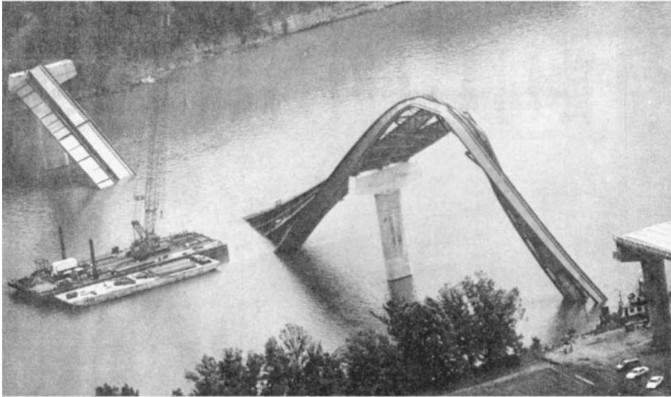
Figure 45.1 Failure of a steel girder bridge during erection, 1995. Steel bridge failures such as this one invite suspicion that the construction engineering aspects were not properly attended to.
