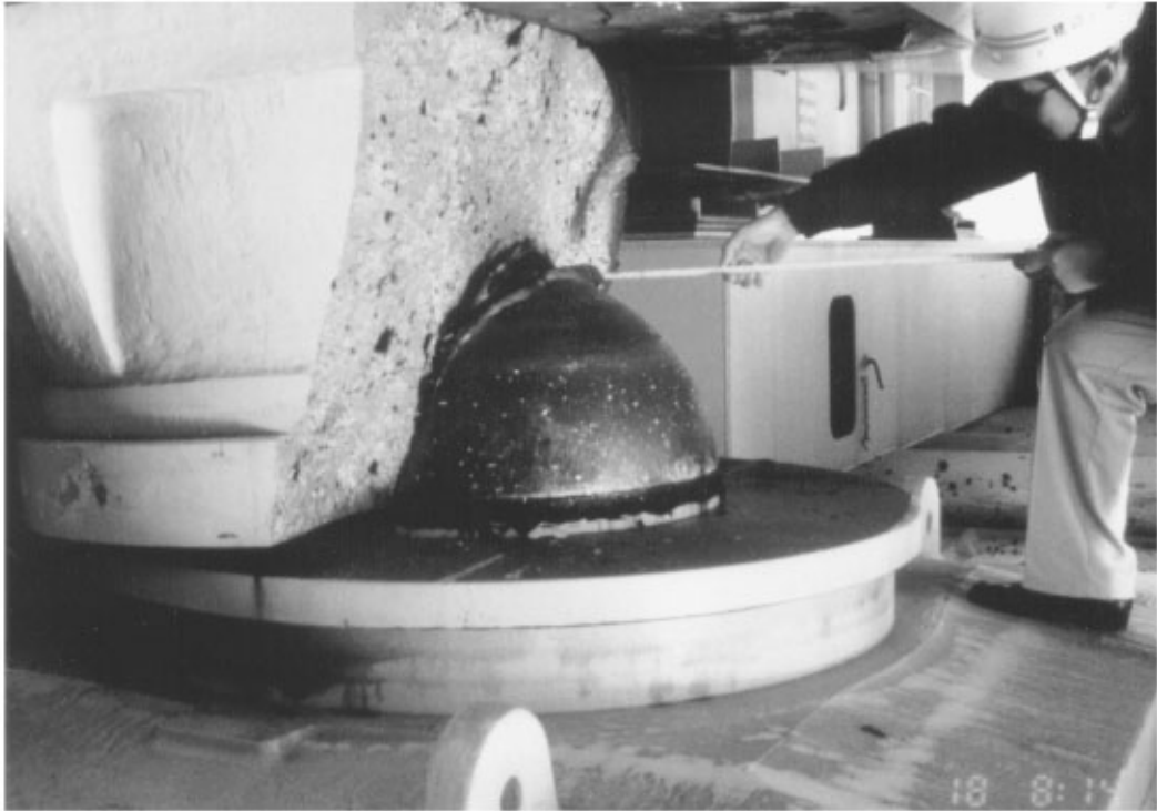
FIGURE 34.16 Nishinomiya-ko Bridge bearing failure in the 1995 Hyogo-Ken Nanbu earthquake.
