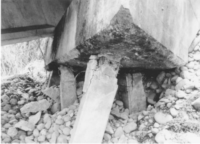
FIGURE 34.33 Abutment piles damaged during the 1991 Costa Rica earthquake. (Source: EERI, Earthquake Spectra , Special Suppl. to Vol. 7, 1991.)
