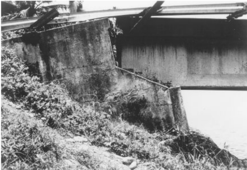
FIGURE 34.32 Rotation of abutment due to liquefaction and lateral spreading during the 1991 Costa Rica earthquake. (Source: EERI, Earthquake Spectra , Special Suppl. to Vol. 7, 1991.)
