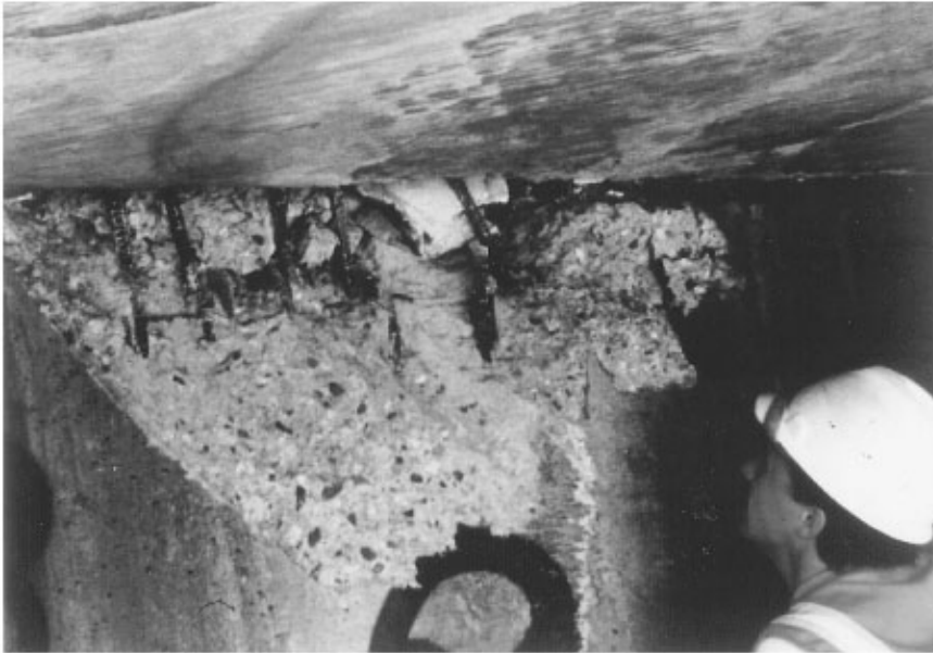
FIGURE 34.31 Damage to internal shear key in an abutment in the 1994 Northridge earthquake. (Source: EERI, Earthquake Spectra , Special Suppl. to Vol. II, 1995.)
