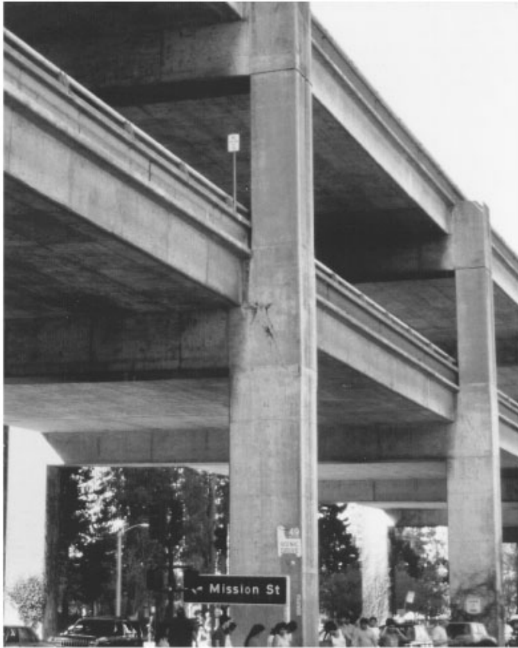
FIGURE 34.28 Embarcadero Viaduct damage during the 1989 Loma Prieta earthquake.
