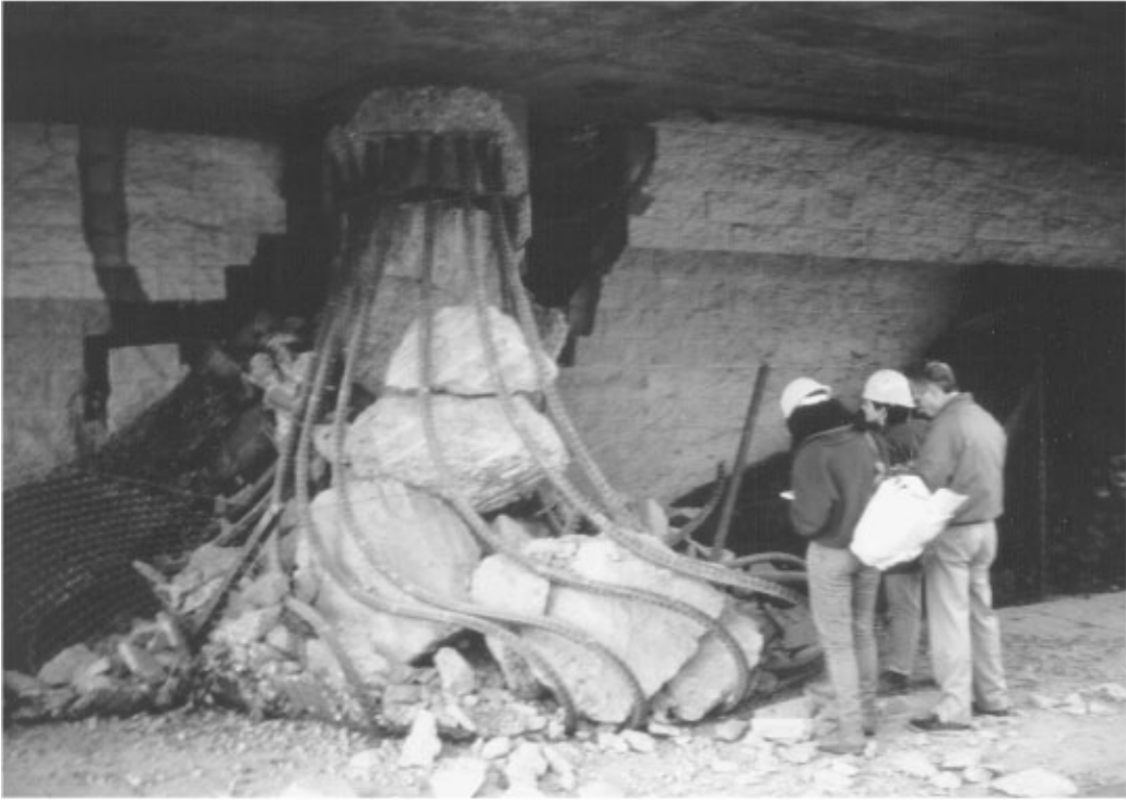
FIGURE 34.21 Failure of columns of Interstate 10, La Cienega-Venice Undercrossing in the 1994 Northridge earthquake. (Masonry walls of storage units are supporting the collapsed frame.)
