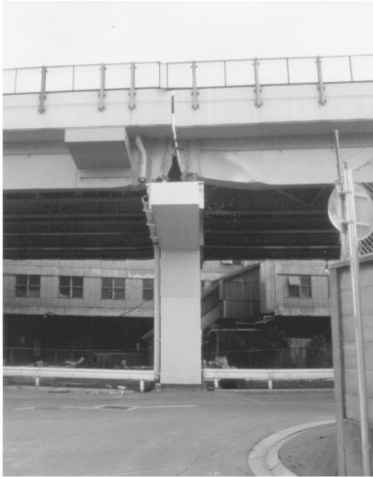
FIGURE 34.13 Girder damage at Bent 351 of the Hanshin Expressway apparently due to transverse movement during the 1995 Hyogo-Ken Nanbu earthquake.
