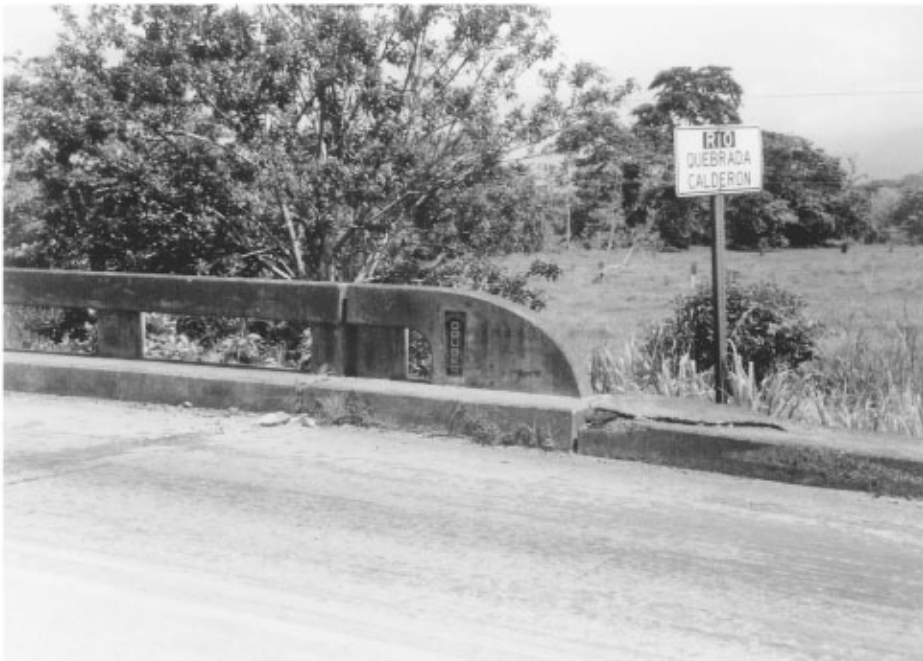
FIGURE 34.34 Settlement slab spanning across slumped abutment fill material at the Rio Quebrada Calderon bridge in the 1991 Costa Rica earthquake. (Source: EERI, Earthquake Spectra , Special Suppl. to Vol. 7, 1991.)
