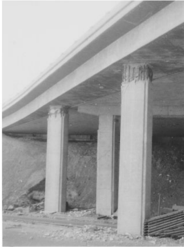
FIGURE 34.17 San Fernando Road Overhead damage in the 1971 San Fernando earthquake.
