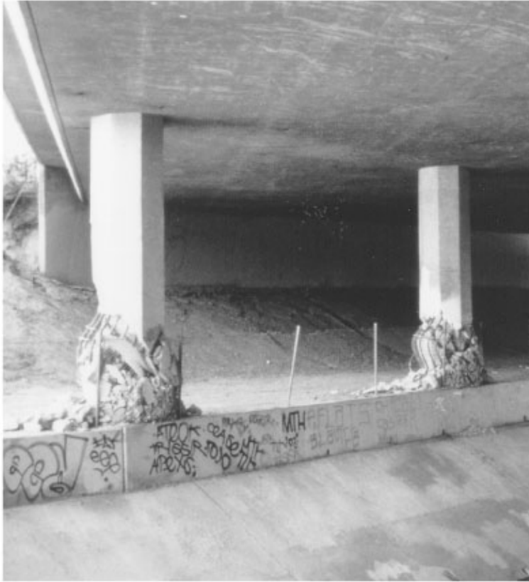
FIGURE 34.5 Bull Creek Canyon Channel Bridge damage in the 1994 Northridge earthquake.
