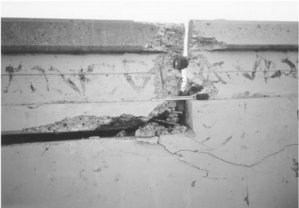
FIGURE 34.11 Santa Clara River Bridge pounding damage in 1994 Northridge earthquake. (a) Barrier rail pounding damage; (b) abutment pounding damage.
