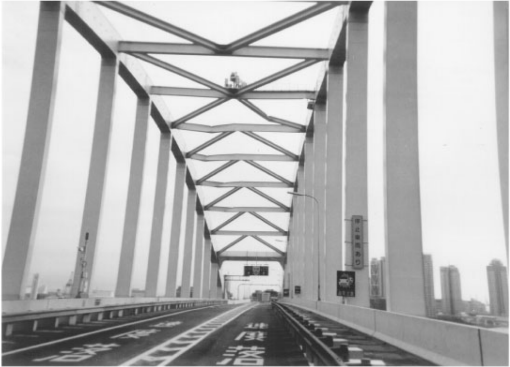
FIGURE 34.14 Buckling of cross-members in the upper chord of the Rokko Island Bridge in the 1995 Hyogo-Ken Nanbu earthquake.
