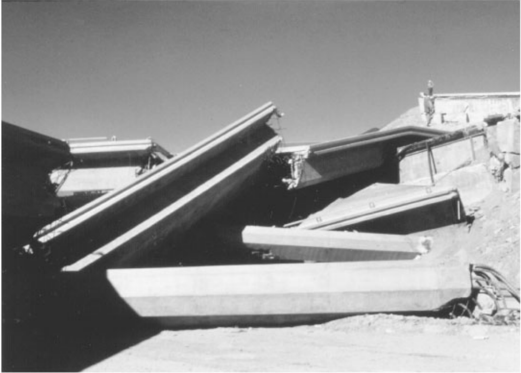
FIGURE 34.24 Failure at the base of a column supported on a single cast-in-place pile in the 1971 San Fernando earthquake [Steinbrugge Collection, EERC Library, University of California, Berkeley].
