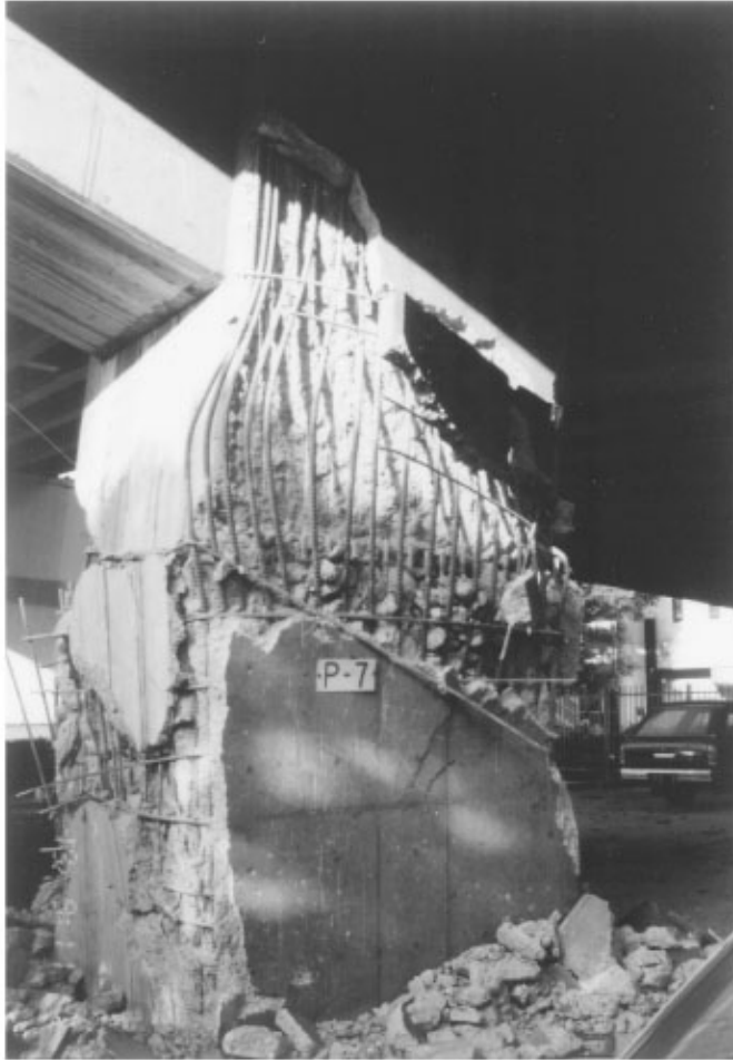
FIGURE 34.19 Failure of column with longitudinal reinforcement cutoffs near midheight in the 1995 Hyogo-Ken Nanbu earthquake.
