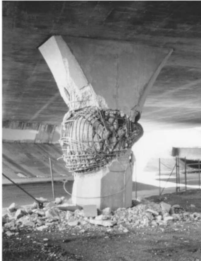
FIGURE 34.22 Failure of flared column in the Route 118, Mission-Gothic Undercrossing, in the 1994 Northridge earthquake.
