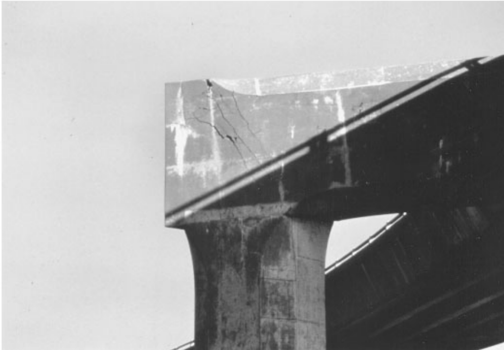
FIGURE 34.27 Outrigger damage in the 1989 Loma Prieta earthquake.
