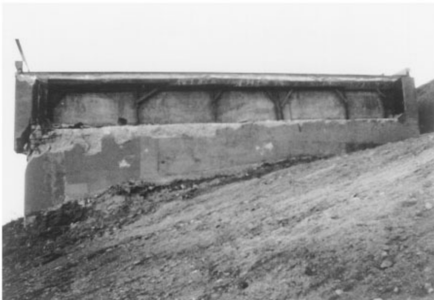
FIGURE 34.30 Damage to external shear key in an abutment in the 1994 Northridge earthquake. (Source: EERI, Earthquake Spectra , Special Suppl. to Vol. II, 1995.)
