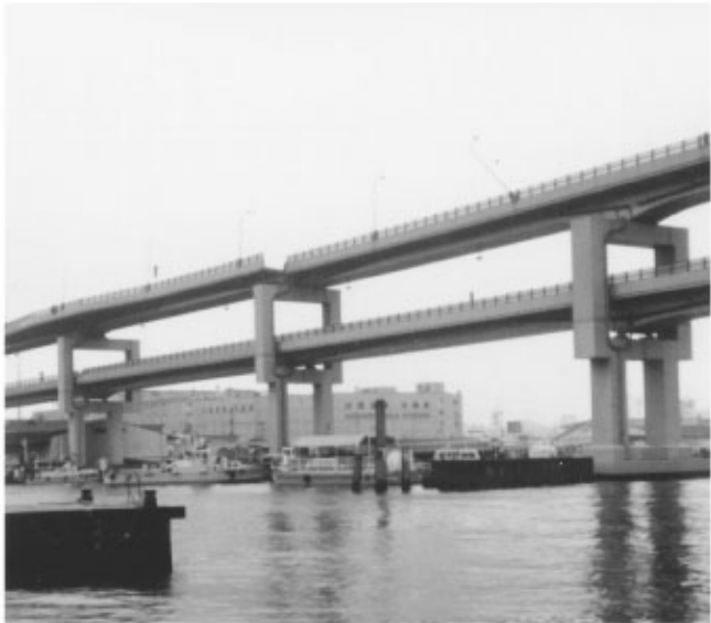
FIGURE 34.15 Hamate Bypass superstructure rotations as a result of bearing failures in the 1995 Hyogo-Ken Nanbu earthquake.
