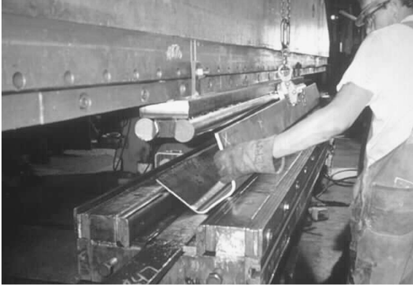
FIGURE 14.2 Press brake forming rib stiffener sections. (Photo by Lawrence Lowe and courtesy of Universal Structural, Inc.)
