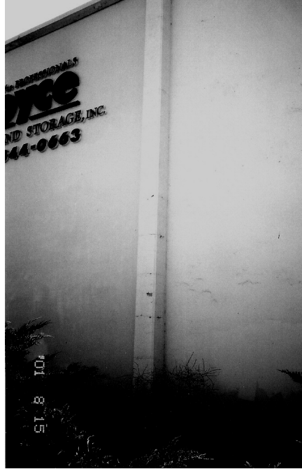
Fig. 4.1 Horizontal cracks in pilaster, north wall
