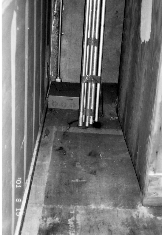
Fig. 3.2 Sensors 1, 11, 12 adjacent to fire wall
