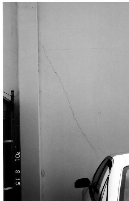
Fig. 4.2 Diagonal shear crack, west wall
