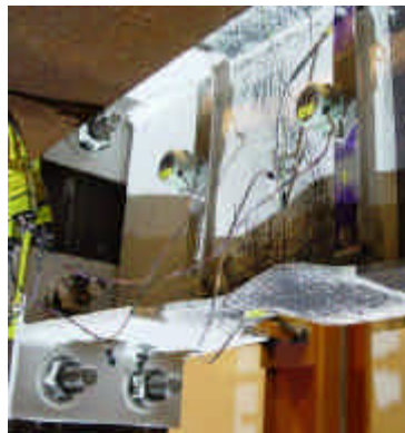
Figure 4.9: 3rd floor beam local buckling after DBE test
