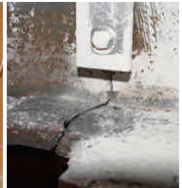
Figure 4.20: Fracture at the 1 st floor north beam
