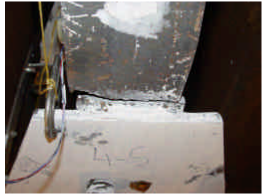
Figure 4.23: Fracture at the 4 th floor south beam
