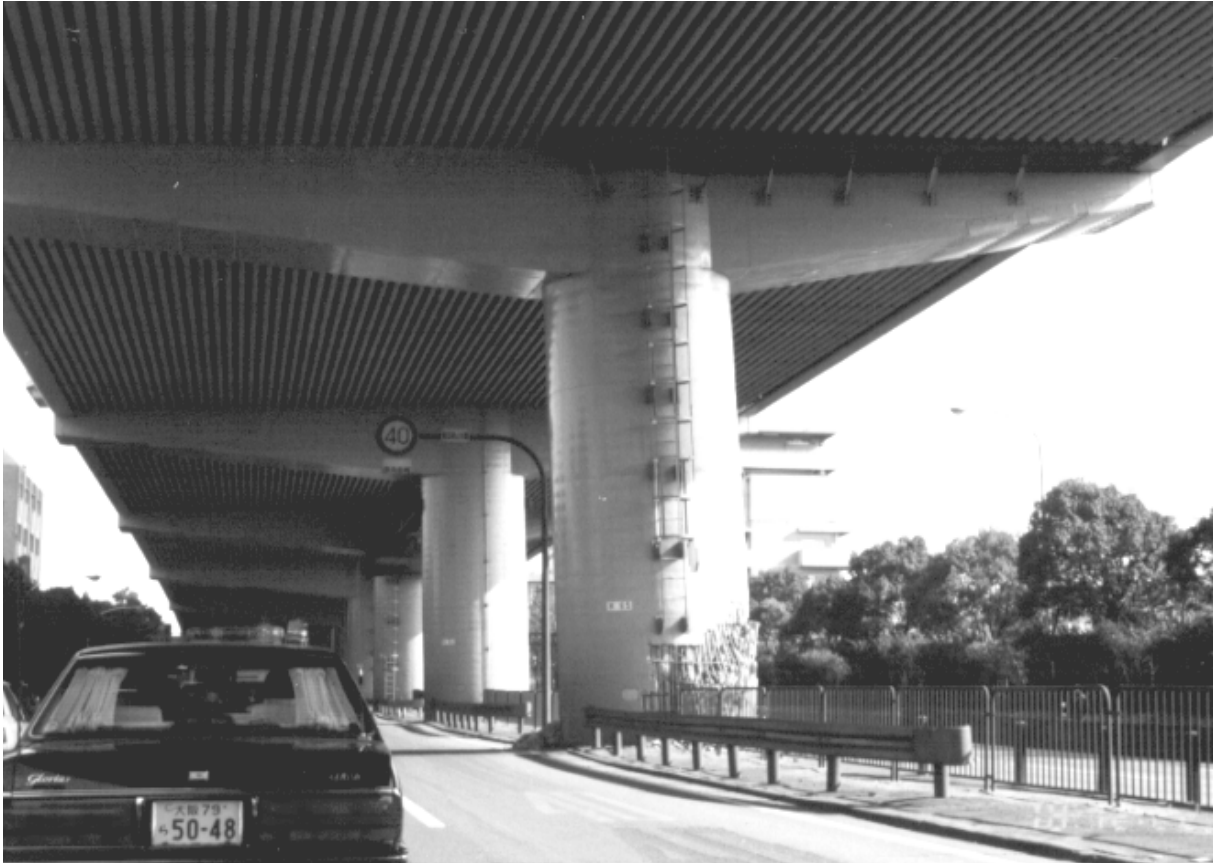
Figure 1.1 A bridge column that suffered large permanent displacement after 1995 Hyogo-ken Nanbu earthquake (Courtesy of Prof. K. Kawashima)
