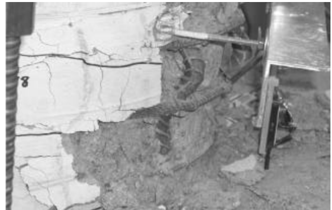
Fig. 17—Buckling of reinforcement in Unit 4.
