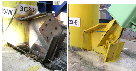
Figure 18. Added stiffeners at the free edges of the gusset at the brace to column joint before Phase-2 tests.
