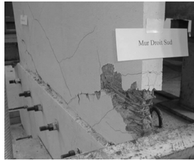
Figure 7. Damage to the edge of the wall at the end of the test sequence (CAMUS 3).
