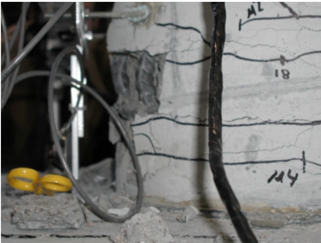
Figure 11.15 North Side of Specimen Buckling
