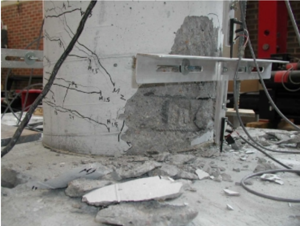
Figure 10.12 South Side of Specimen at Ductility 6
