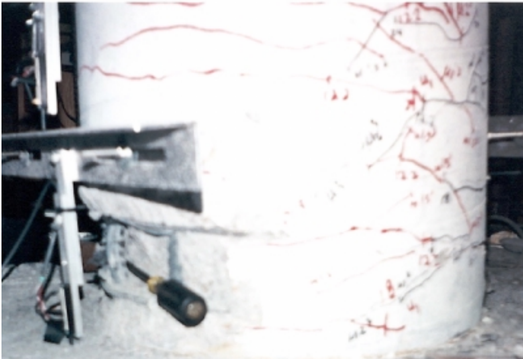
Figure 8.9 Buckling of Reinforcement South Side of Specimen at Ductility 4
