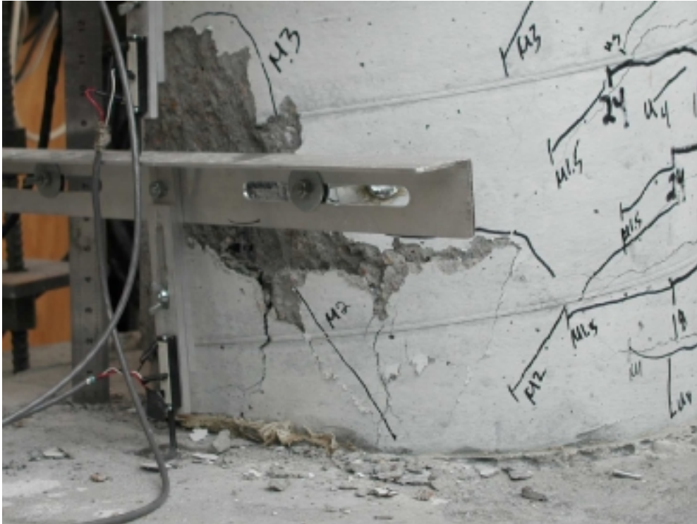
Figure 10.8 South Side of Specimen at Ductility 3
