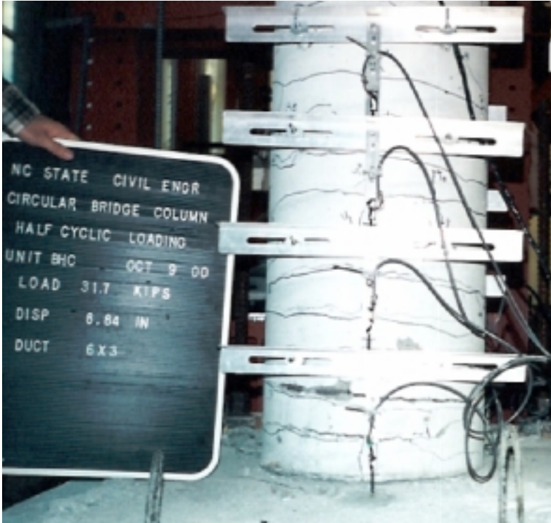
Figure 9.11 North Side of Specimen at Ductility 6 Cycle 3
