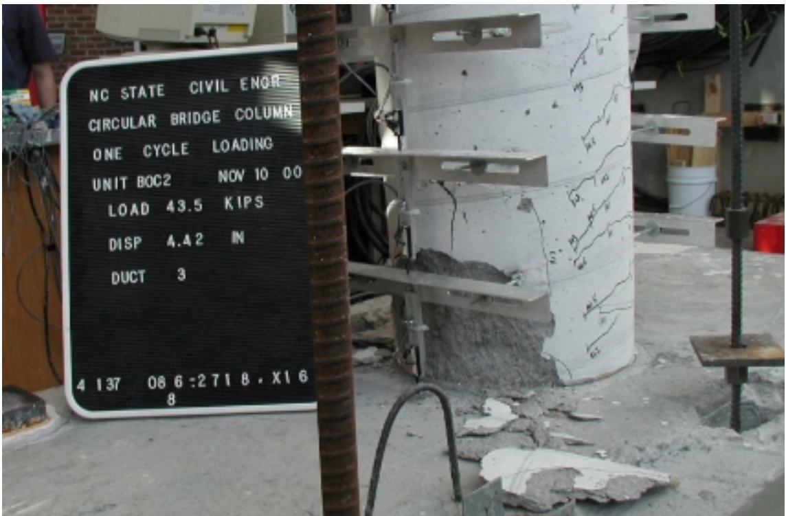
Figure 11.7 South Side of Specimen at Ductility 3
