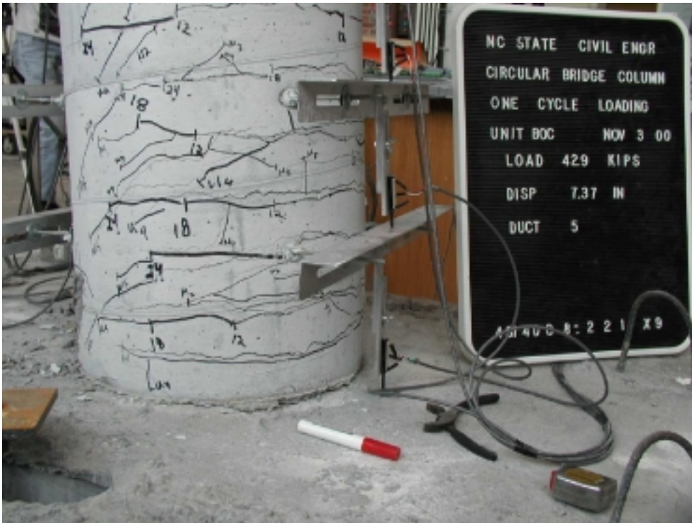
Figure 10.10 North Side of Specimen at Ductility 5
