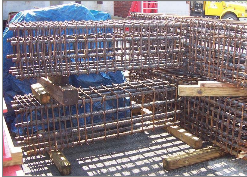
Figure 3.8. Reinforcement Steel - Ductile Shear Failure Specimen (Top), Brittle Shear Failure (Bottom)
