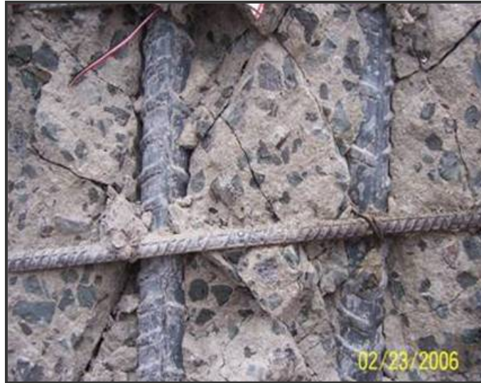
Figure 1.1. Lightweight Concrete Fractures
